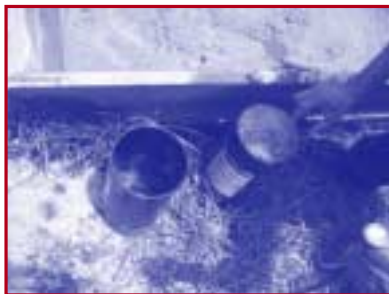
Poor quality concrete in Boaco
