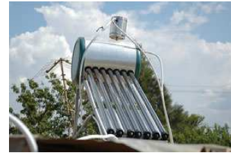
A solar water heater on the roof of a house. The water is in the tank. 5
