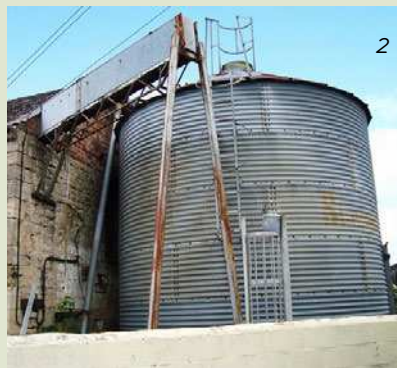
A tank made from corrugated iron.
