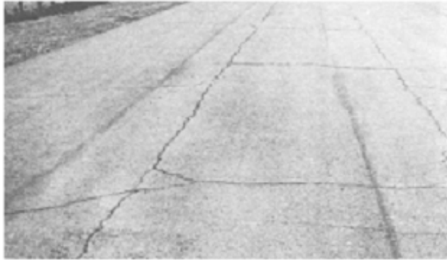
Figure 6.2: Typical block cracking due to shrinkage
